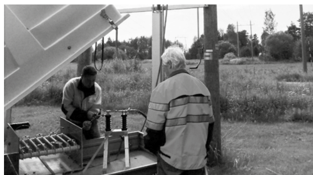
The algorithms have been proven effective in extensive field tests with electrical utilities, and have been installed in networks since 2014.
