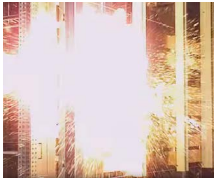
Level of damage
