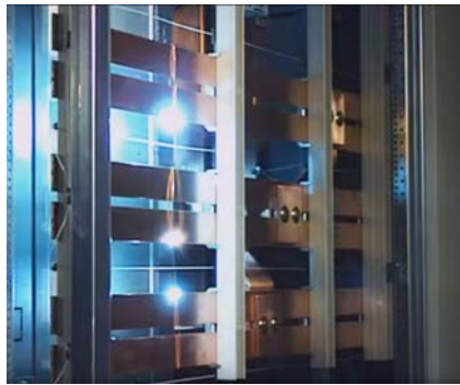
Level of damage
